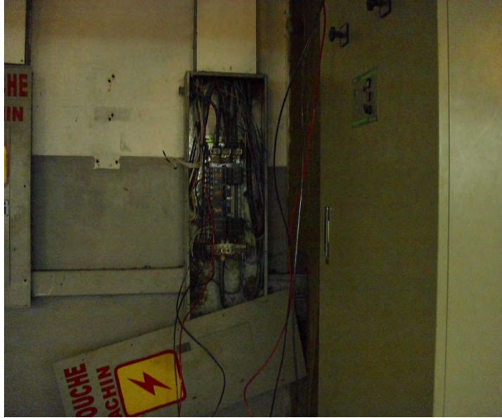
Figure 1. This electrical panel represents a possible ignition source as well as a potential source of shock or electrocution to workers.
